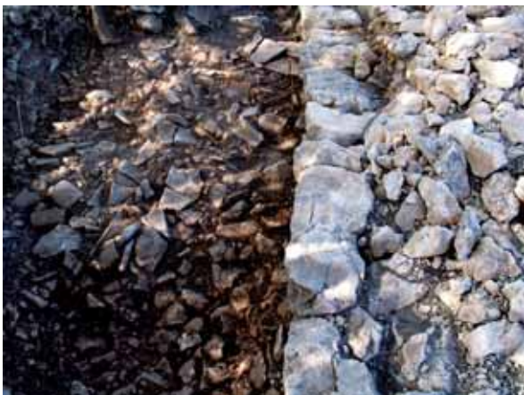
Fig. 8 Part of the western wall of the castellum with tegulae fallen from the roof of the adjacent portico
